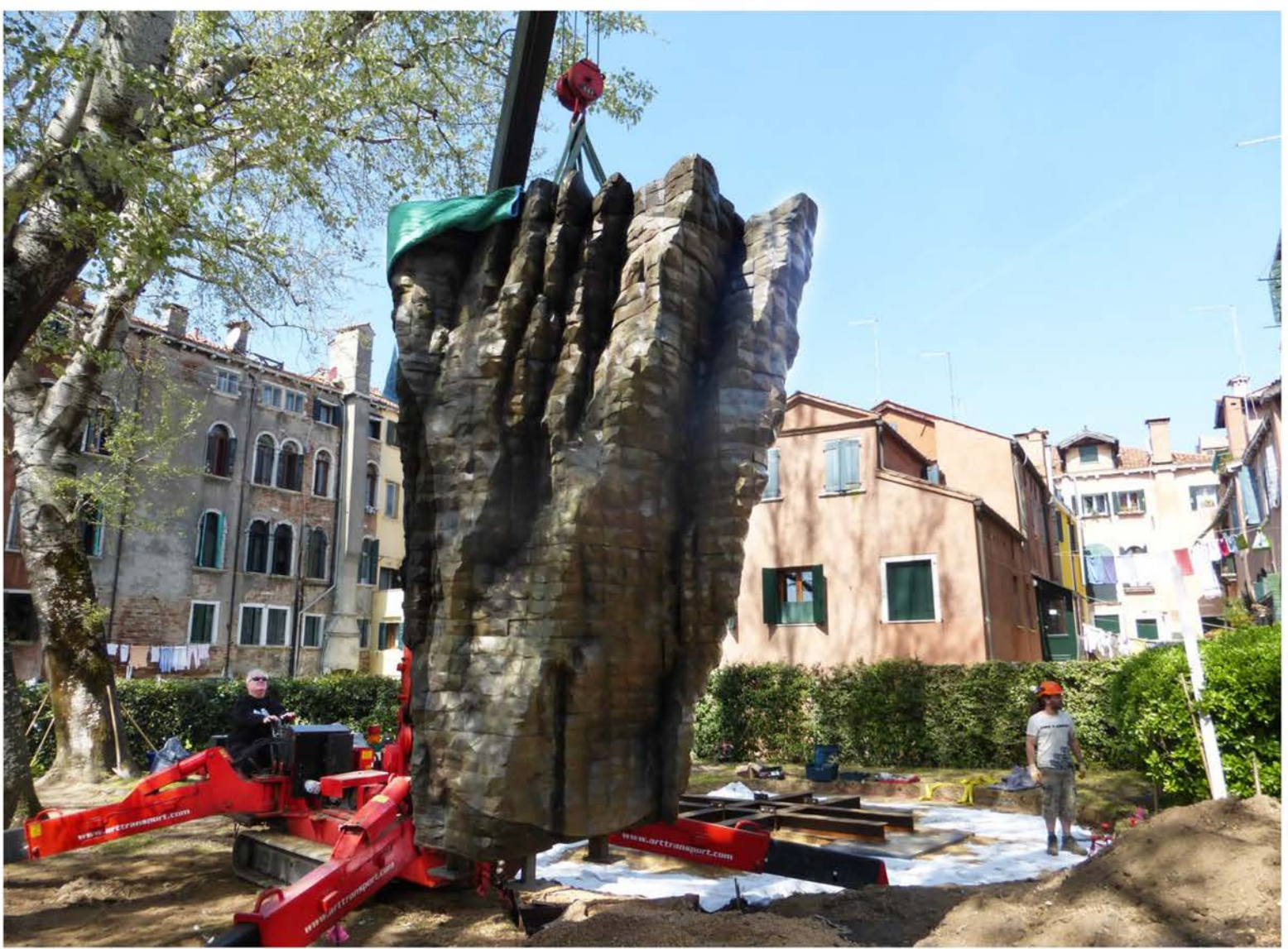
Lowering a sculpture into place. The sculptures required more than 12 tons of steel armature underground for support. Source: Yorkshire Sculpture Park via Bloomberg
